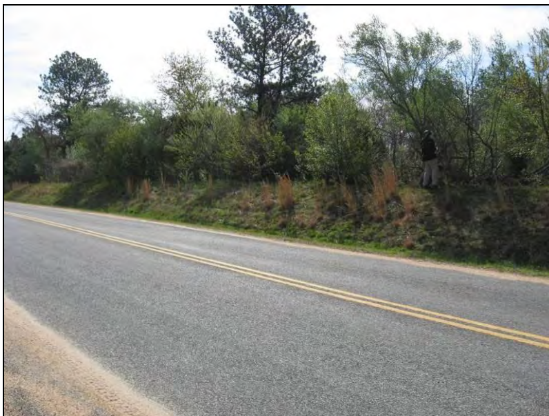
Photo 6: View of Earthen Berm Located Along the I-64 Corridor at the Western End of the Survey Area, Facing Southeast Across Woodview Drive.
