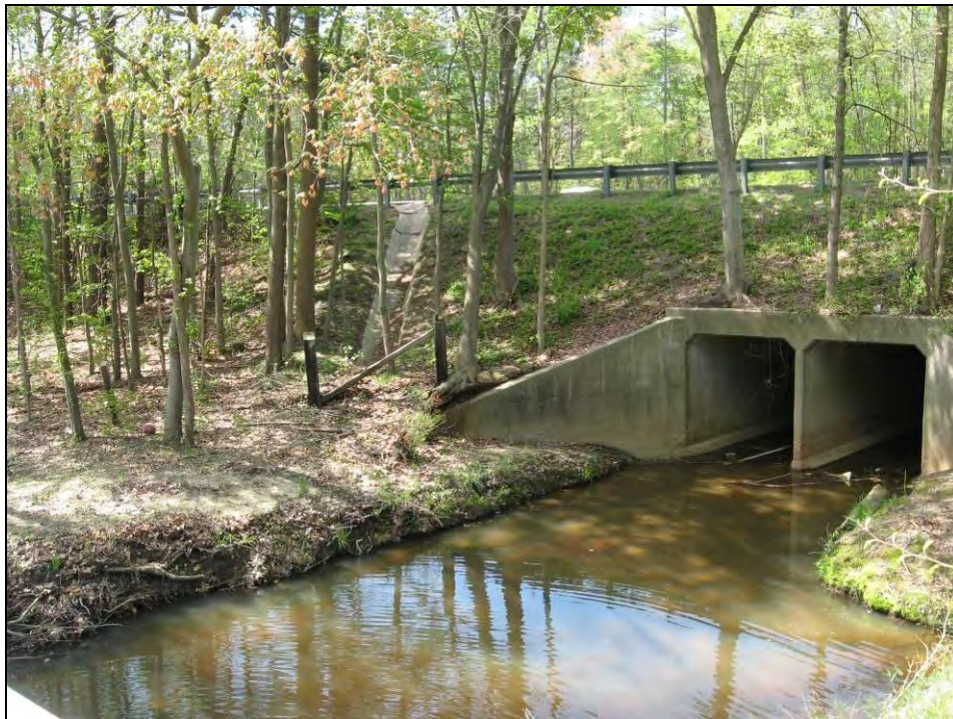
Photo 33: Overview of Concrete Culvert and Drain in the Survey Corridor, Facing West.
