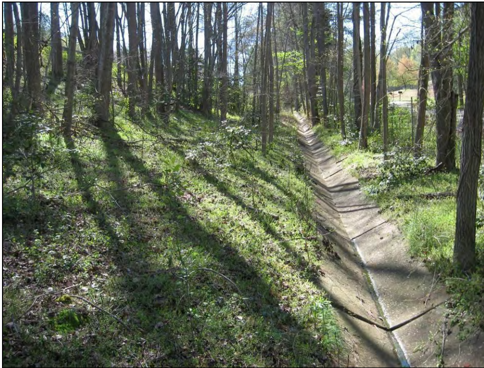
Photo 9: View of Cement Drainage Channel Located at the Western Edge of Site Boundary, Facing West.
