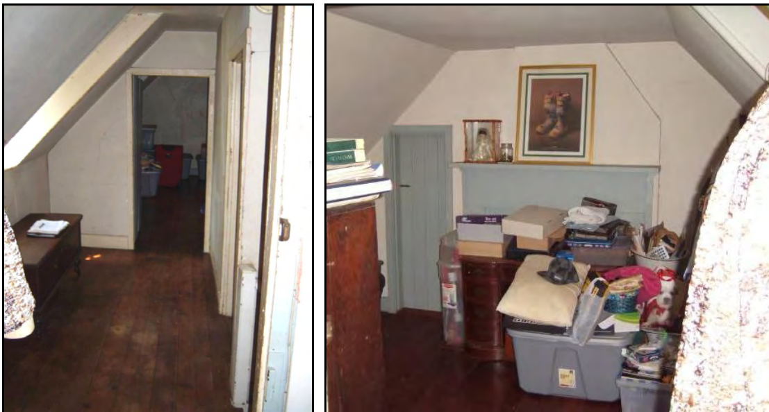
Photo [GROUP] 12: [LEFT] View Towards West-End Bedroom from Hallway on Second Floor; [RIGHT] View of East-End Bedroom on Second Floor (Dovetail, Sep. 2011). NOTE: Door in upper-left corner opens into a closet in the two-story side addition.
