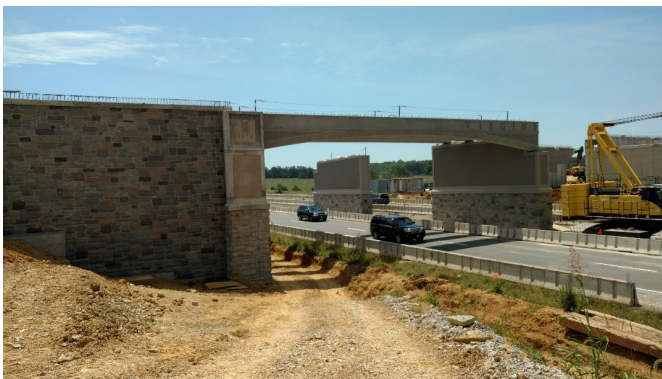
Branch's Southgate project is an at-grade intersection being improved to a grade-separated DDI in Blacksburg, VA.
